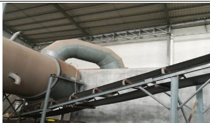
热风烘工序废气三级沉降除尘
