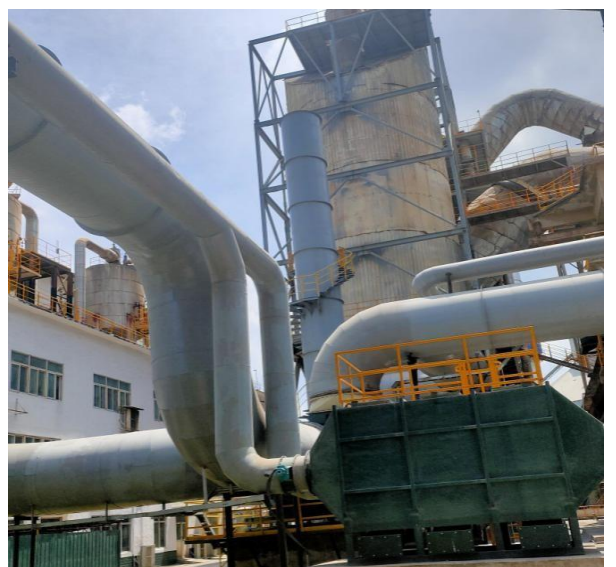
1#危废车间废气排气筒
